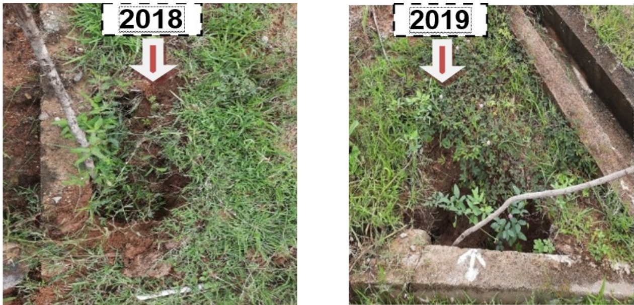
Fig. 4. Sinkhole formation on the downstream slope of the dam during 2018–2020
