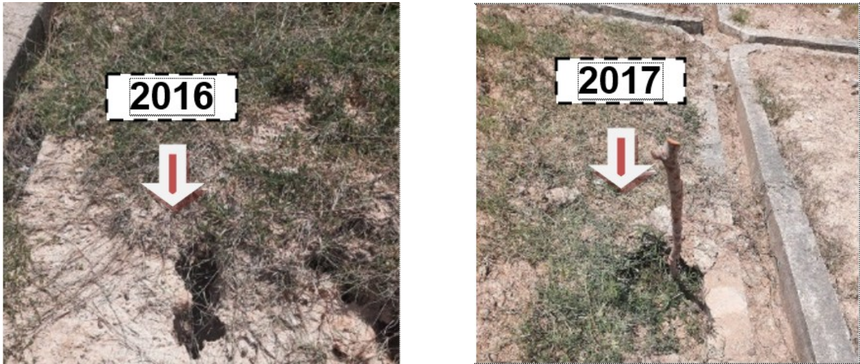
Fig. 3. Sinkhole formation on the downstream slope of the dam during 2014–2017
