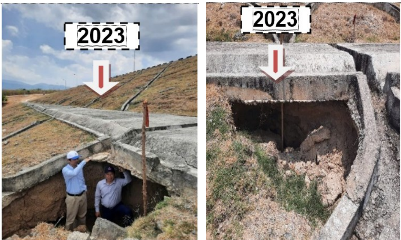
Fig. 5. Sinkhole formation on the downstream slope of the dam during 2020–2023
