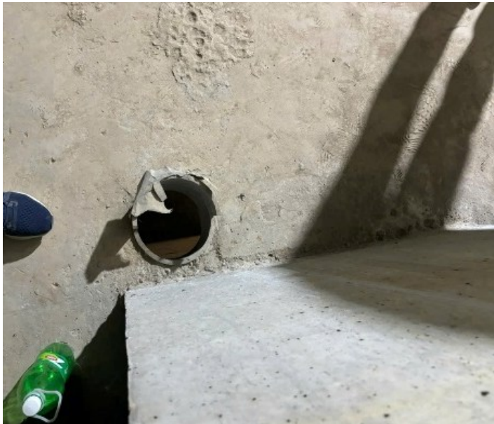
Fig. 1. Circular openings adjacent to the column
