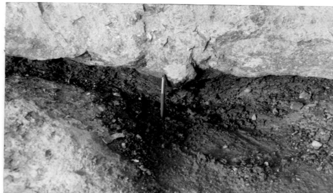
Fig. 3. Weathered Rock Seam developed along the contact of two flows (Adopted from [10])
