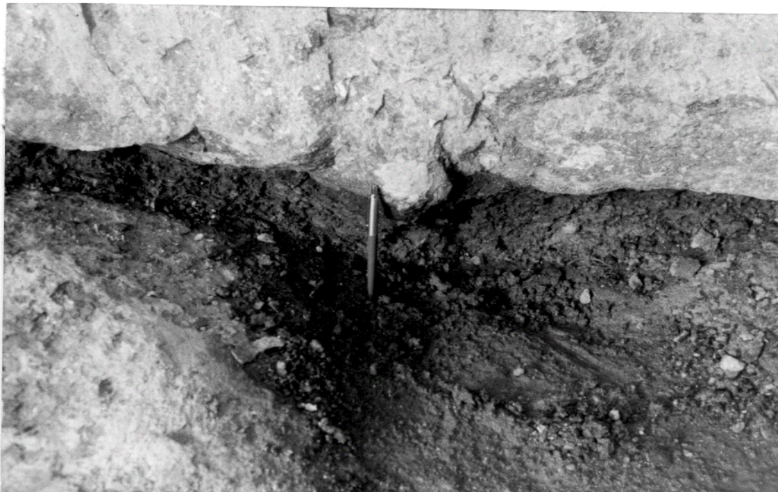
Fig. 7. Weathered rock seam developed at the contact of basalt flows in the foundation of Karjan dam [14]
