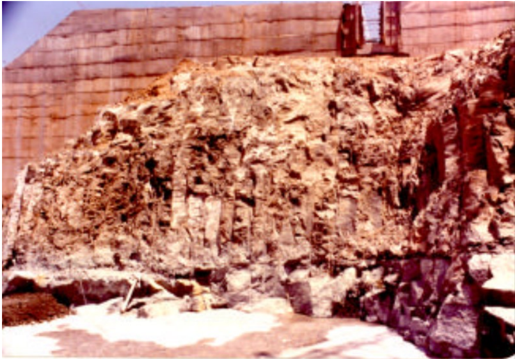
Fig. 6. Treatment of intra-formational shear associated with red bole layer in the spillway foundation of Narmada Dam [14]
