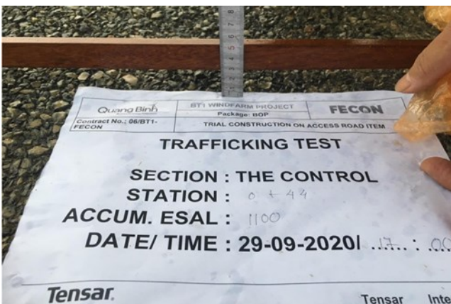
Figure 7. Measure of rutting depth
