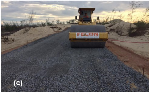
Figure 3. Construction process of trial unpaved road (a) subgrade preparation; (b) Subbase & base preparation; (c) Base compaction
